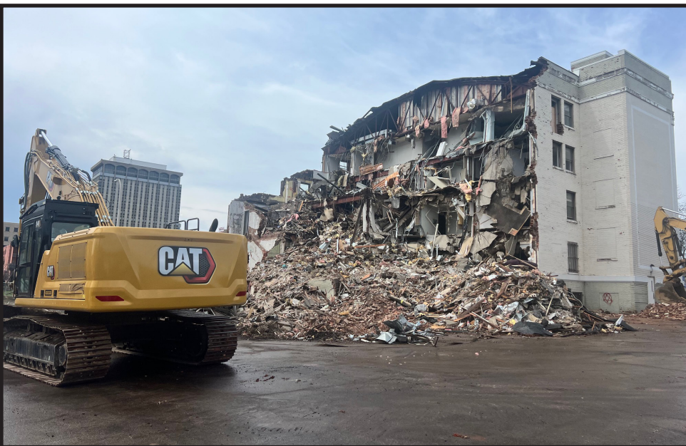
The Peoria Labor Temple, that housed labor for almost 100 years, is being demolished to make way for a veterans homeless shelter. The contractor on the project is River City Demolition.
